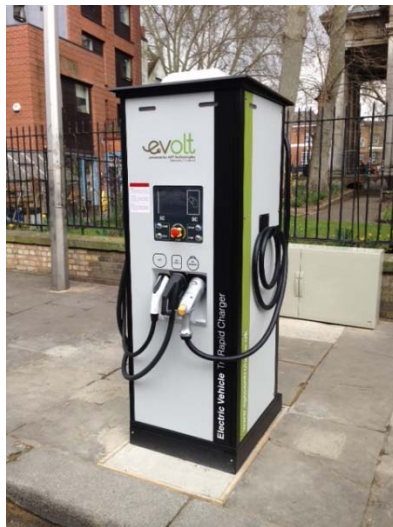
Newly installed EV charging point near taxi rank at Calvert Avenue
